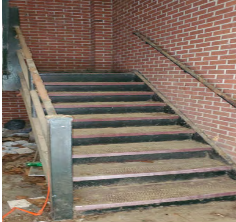
Photograph 5 - Typical Lead-Based Paint on Stair Components (Railings, Risers, Stringers, etc.) of Vance Hall.
