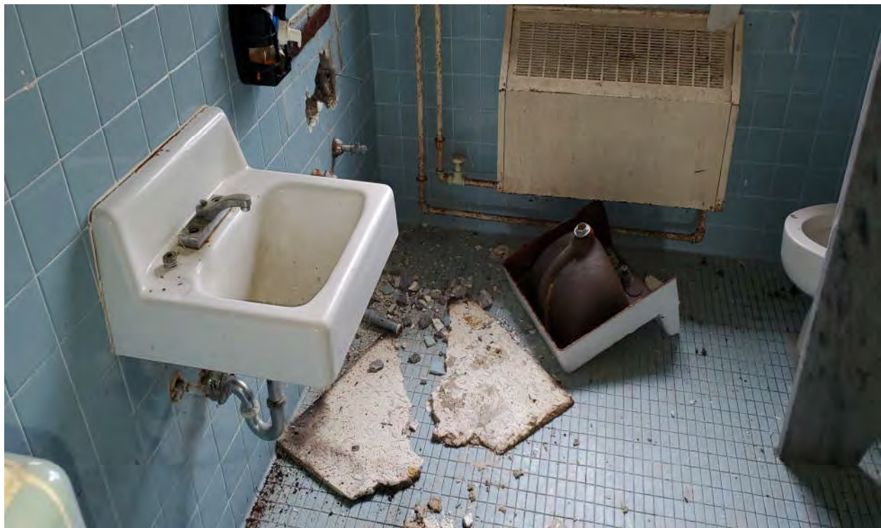
Photograph 6 - Typical Lead-Containing Coating on Porcelain Sinks Located Throughout Vance Hall.
