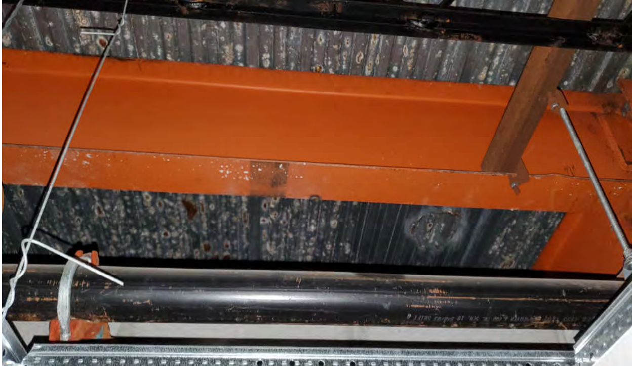
Photograph 3 - Typical Lead-Based Paint on Metal I-Beams Located Throughout Bryant Hall.
