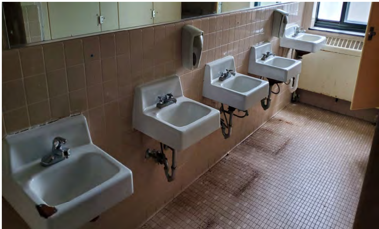
Photograph 2 - Typical Lead-Containing Coating on Porcelain Sinks Located Throughout Bryant Hall.
