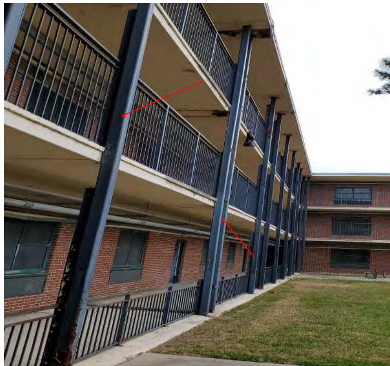
Photograph 4 - Typical Lead-Based Painted Support Columns Located Throughout the Exterior of Vance Hall.
