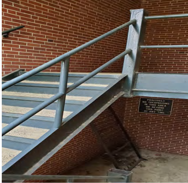
Photograph 1 - Typical Lead-Based Paint on Stair Components (Railings, Risers, Stringers, etc.) of Bryant Hall.
